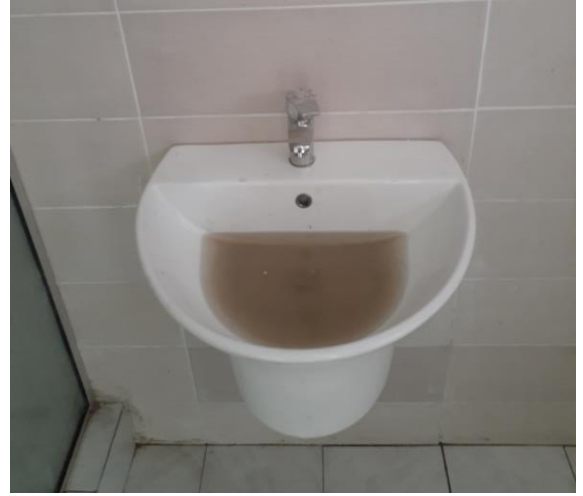
Clogged basin in Bedroom 3
