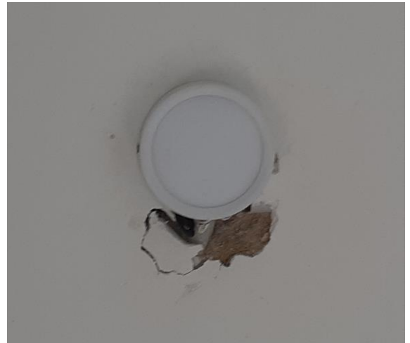
A crack around the ceiling mounted LED light in the Maid's room (needs little rectification).
