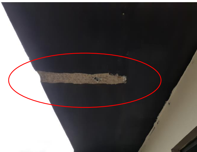
Slab chiseled on the balcony accessible from the family lounge (would need to be plastered and painted).
