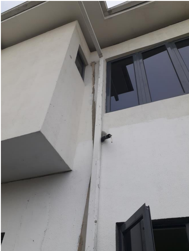
Poorly anchored roof gutter
