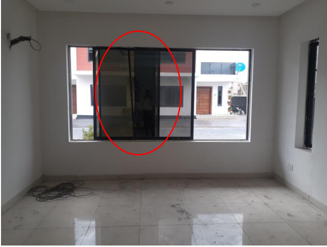
A broken window pane with a bad frame in the Living room
