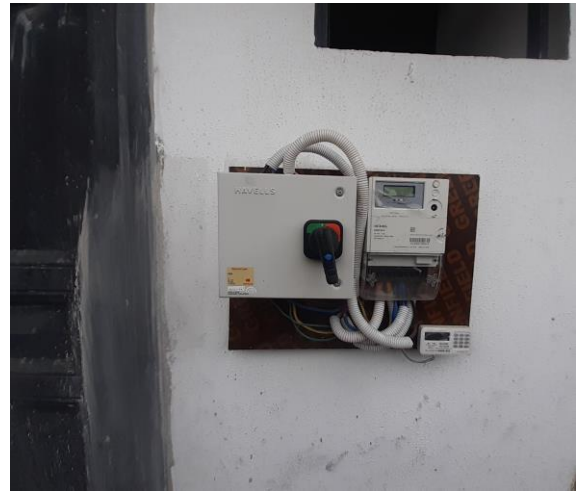
Smart meters have been preinstalled
